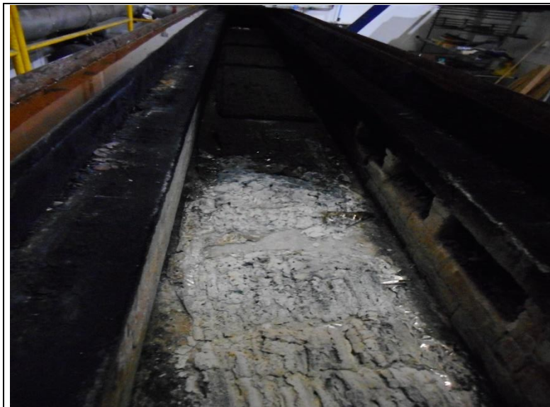
Photo No. 2 Post Test
